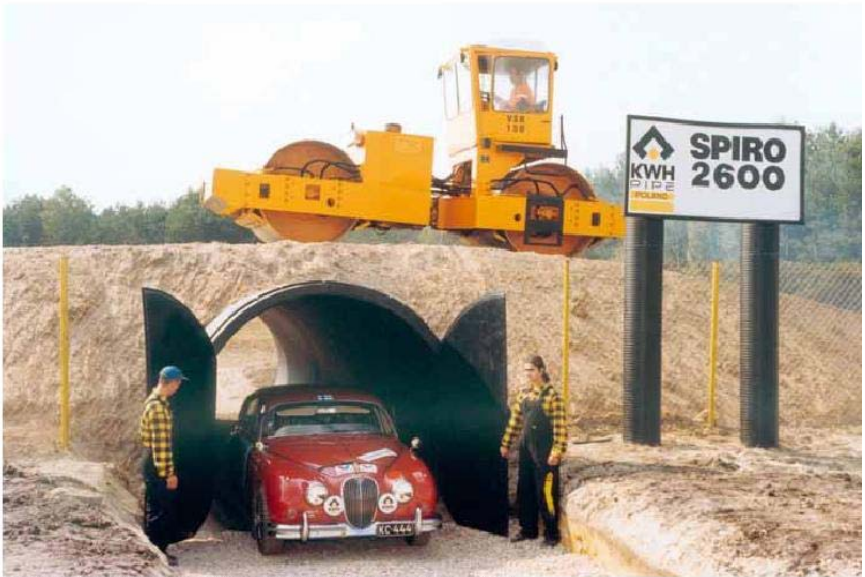
Pict 6.1.a. 17 caterpillar, 0,5m of cover. No deflection is visible. Pipe stiffness is 2\text{kNm}^2 .
